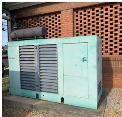
Existing Cummins Onan 100ENBA Generator
