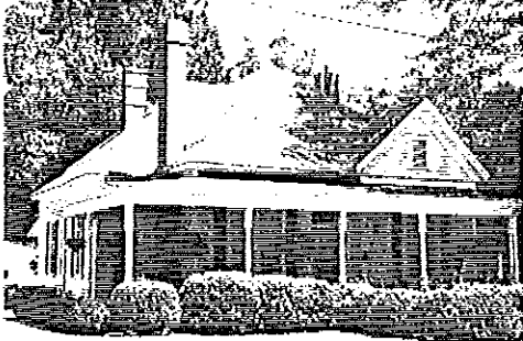
The built-in box gutter located along the porch cornice of this structure is a typical type found in the district.
