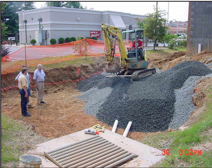
Conversion of a small-scale sediment trap to bioretention. The photos shows adding an underdrain system.
