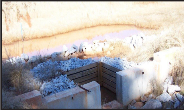
Example of Slotted Board Dam
