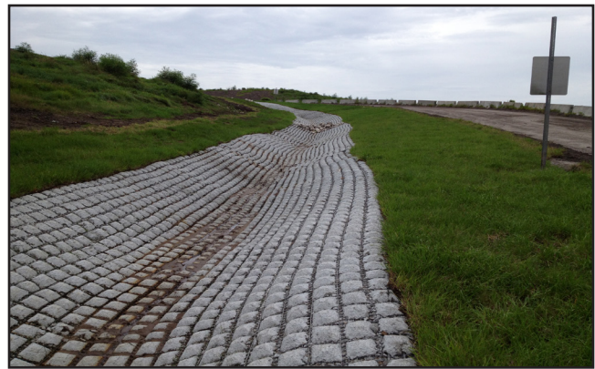
Figure 2.9- This vegetated waterway will safely convey storm water away.
