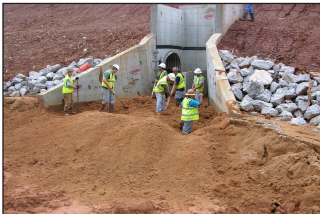
Figure 1.2 - Maintaining outlet protection due to BMP failures higher in the drainage basin.
