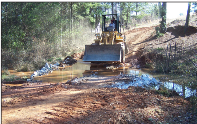
Figure 2.14 - Temporary bridges or culverts should be employed when construction equipment is required to cross natural or constructed channels
